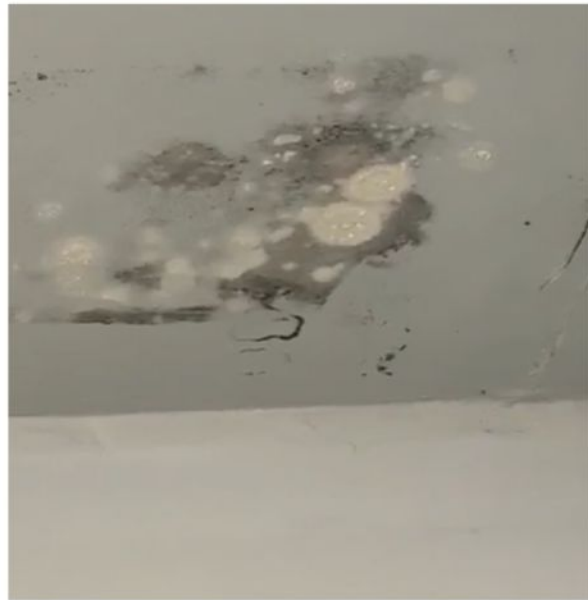
Mold spores blooming on the ceiling of the workers' bathroom, Jun. 2020
